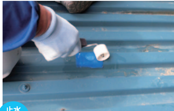
止水 Water stop 折半屋根の漏水補修 Corrugated roof water leakage repair
