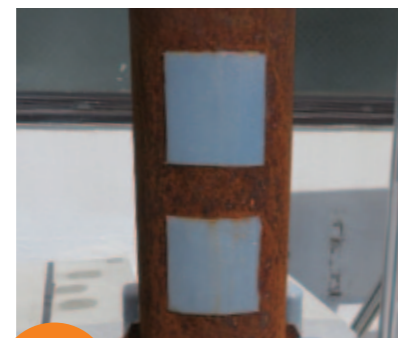
防食 Anti-corrosion 鋼管柱の表面防食 Corrosion protection of steel pipe columns
